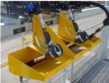
Pictured: “Drip trays” at Oakland, CA facility
